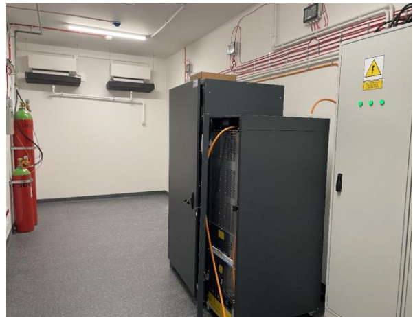
Server room in Stage 3A
