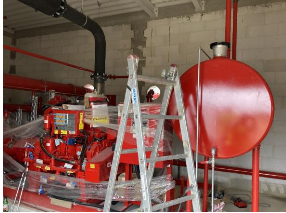
Technical area - pumping station
